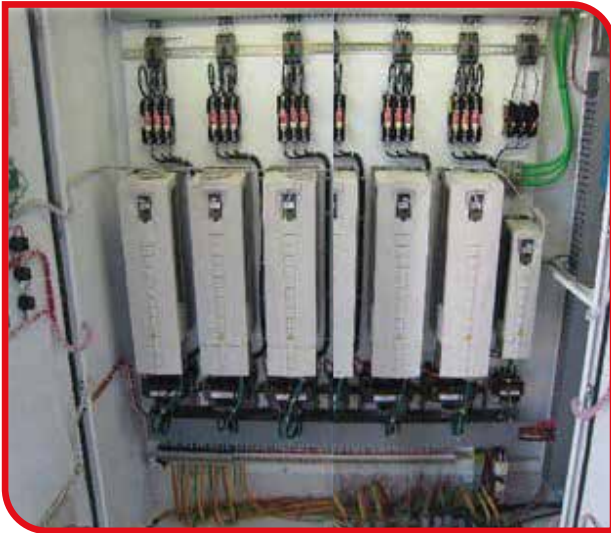
VFD (VARIABLE FREQUENCY DRIVE)
